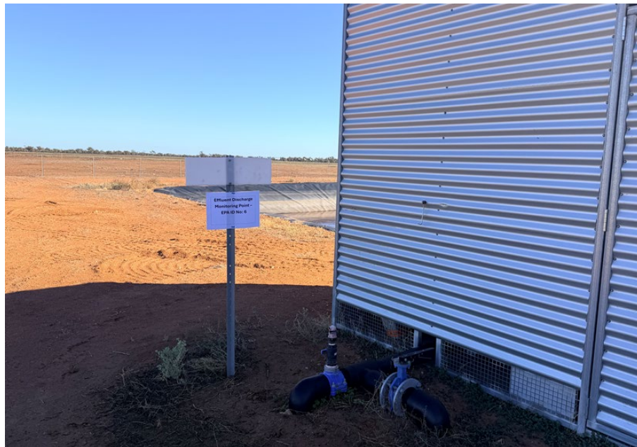
Effluent discharge Point 6 monitoring location
