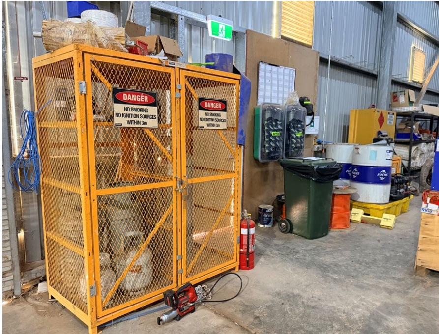
Class 3 Gas storage with combustible on top, no placard, Lithium-ion battery powered compressor out front, and insufficient segregation from Class 3 Flammable Liquids.
