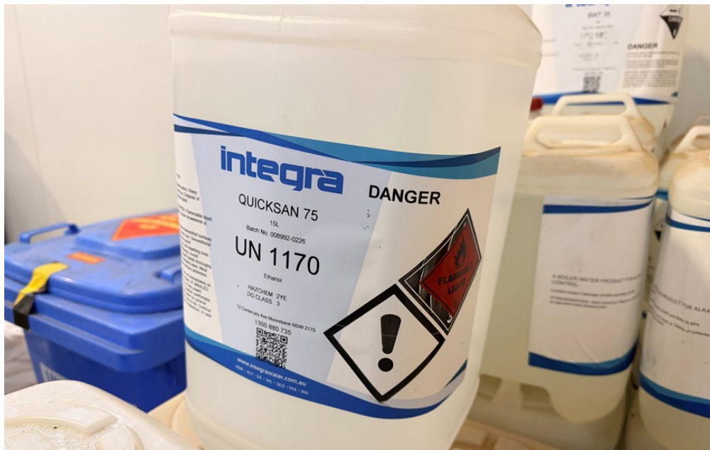
Class 3 Flammable Liquid and Class Corrosive stored together without segregation in the Main Chemical Store room. No placard on door.
