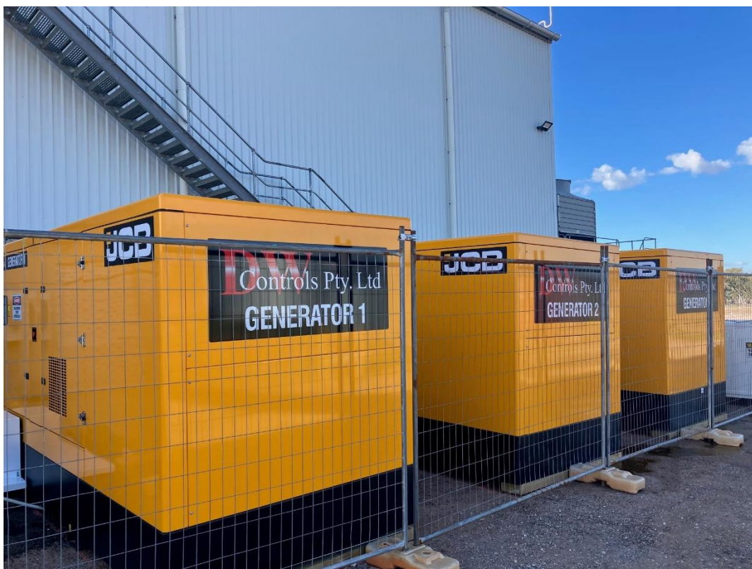
Figure 11: New generators onsite
