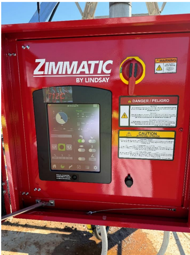
Figure 20: Center Pivot Control Panel
