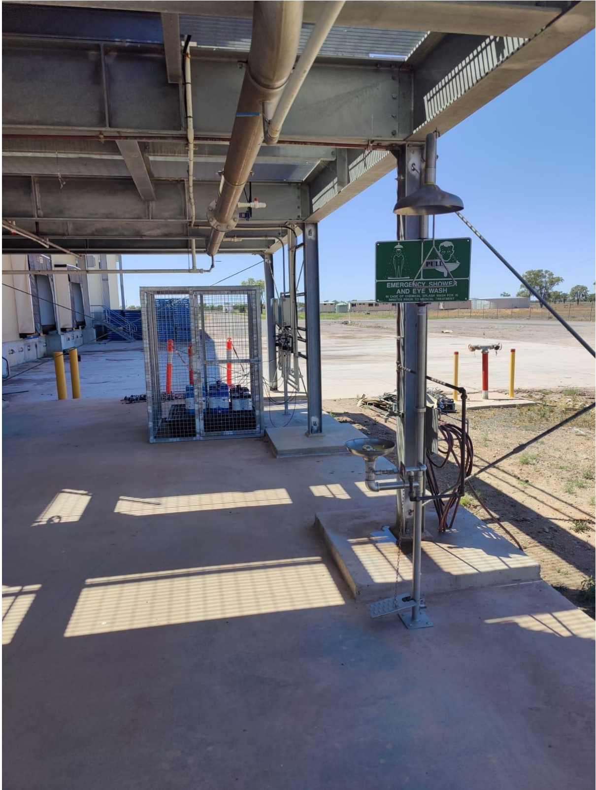
Figure 12: Water dosing chemical stored on a bunding
