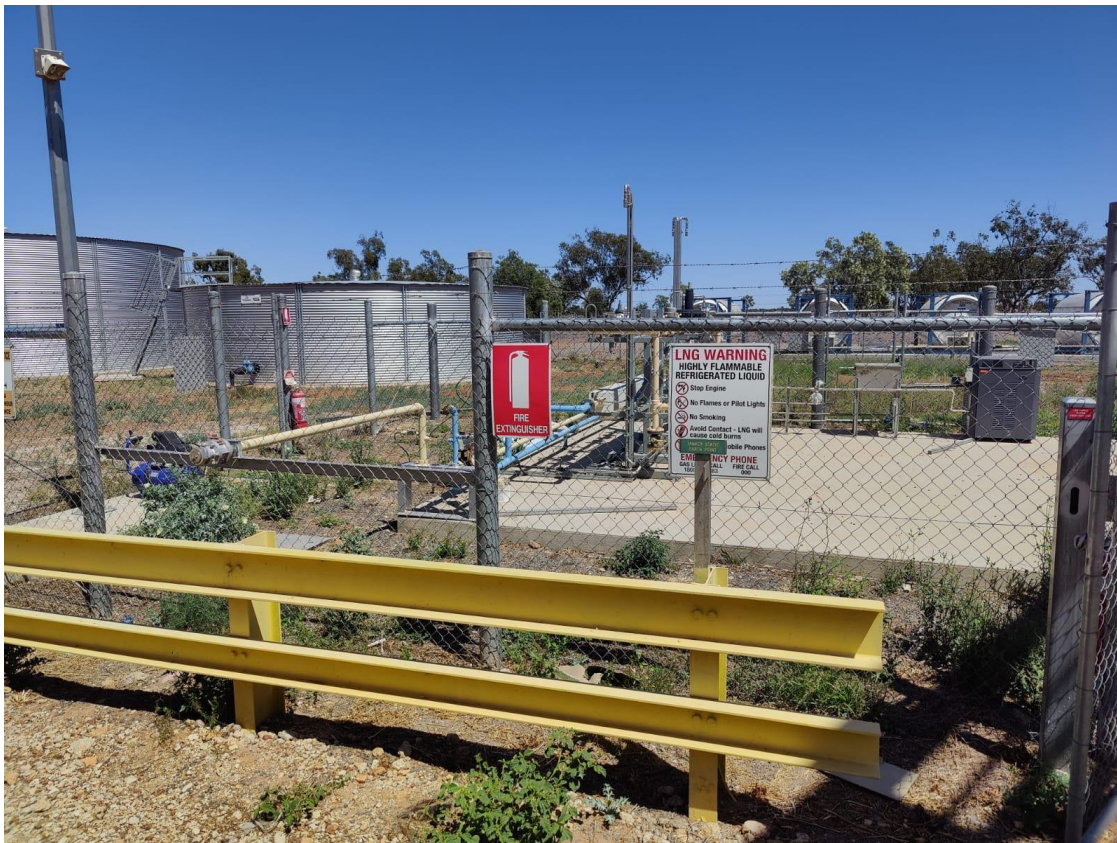
Figure 11: Safety Signs for LPG filling area
